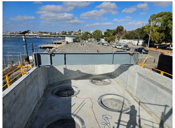
Figure 3: View inside the pile cap shell – the 'circles' are pile 'cut outs'
