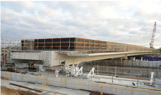
The Stirling Station Bus Bridge laterally slid into place over Mitchell Freeway.
